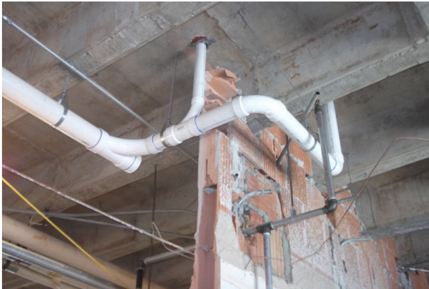
Fire Caulked Plumbing to 5 th Floor
